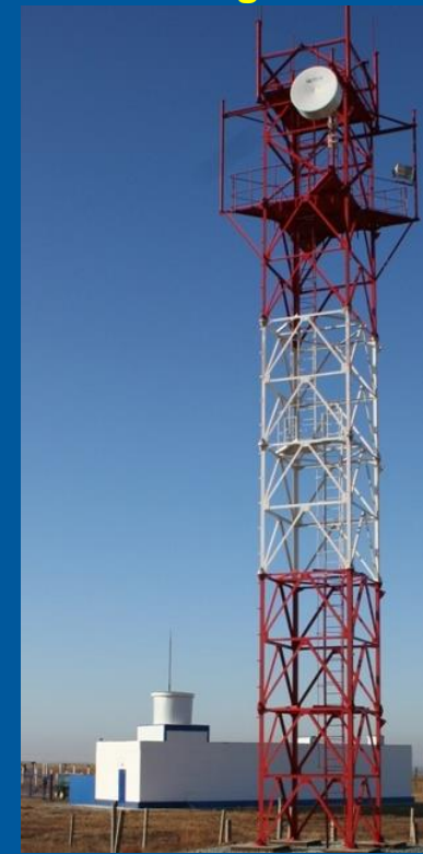
Set of Telemetry, Data Collection and Processing means
