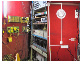
Old & new electrical installation
