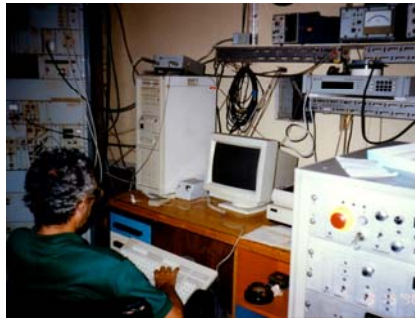
Control room circa 1994
