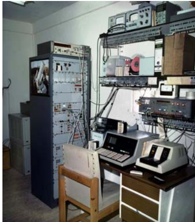
Control Room circa 1985
