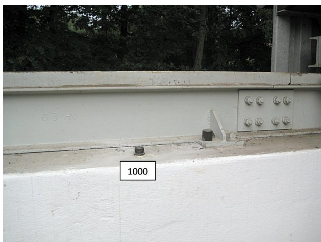
Figure 2 Marker 1000 on wall crest in building A 11
